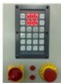
24V Control panel
